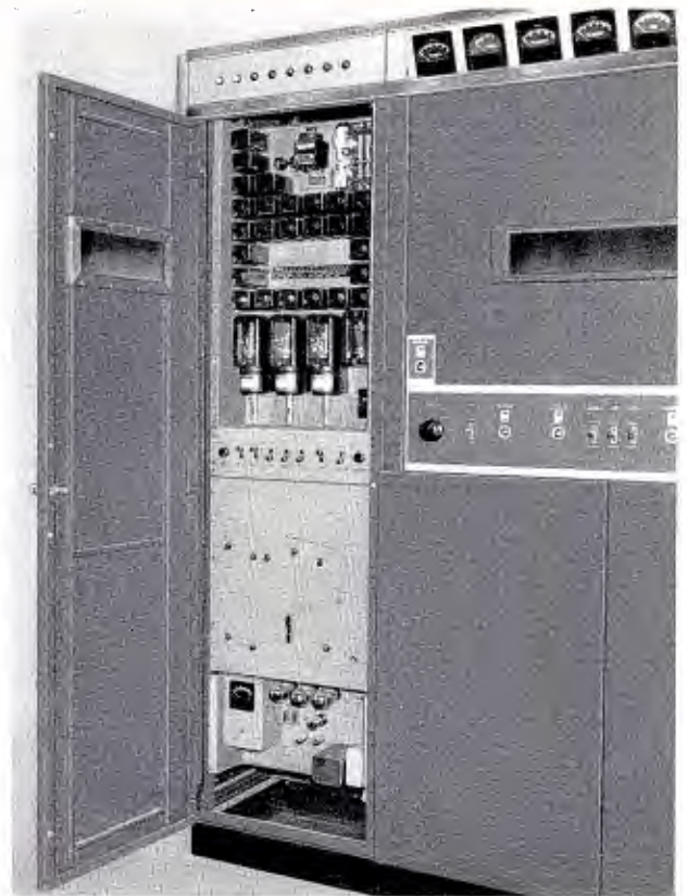
Control circuits of the TT-6AL are grouped in separate cabinet with status lights on a panel above the door. Auxiliary switches, breakers, overload and auxiliary relays, and overload indicating lights are located behind door.
