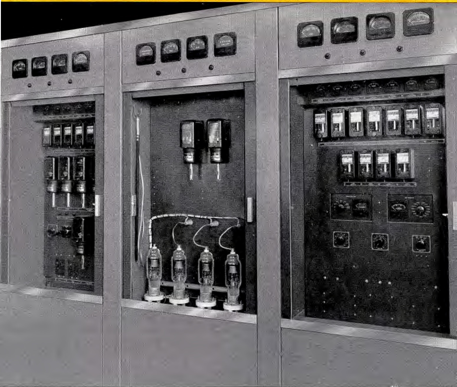
Central cabinets of the 10 kw driver showing control and distribution, screen rectifier, and regulator units.
