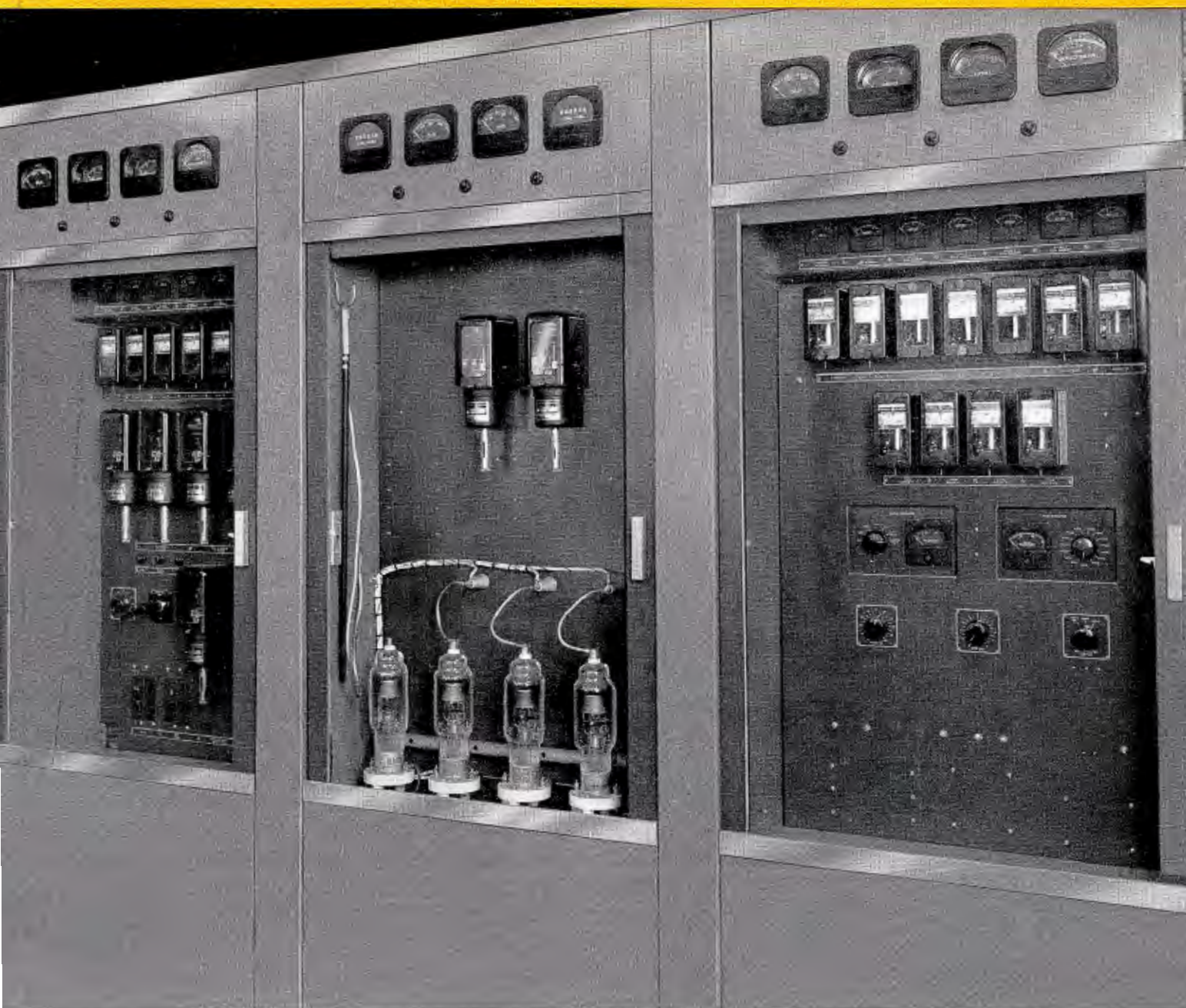
Central cabinets of the 10 kw driver showing control and distribution, screen rectifier, and regulator units.
